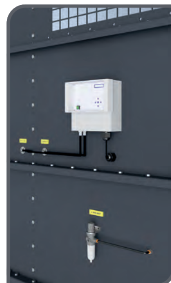
Differential Pressure Pulse Control Unit and Compressed Air Connection
