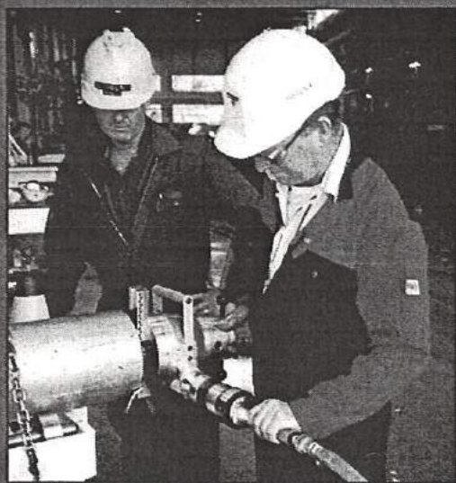
Solution Profile: The handy Model 212B BEVELMASTER™ on the job performing a weld preparation bevel on stainless steel pipe.
