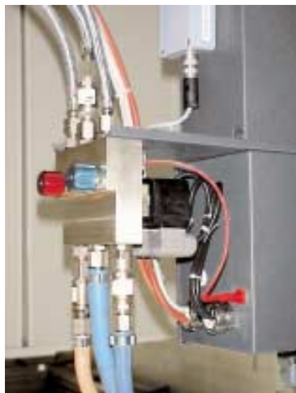
Valve block and proportional valves
